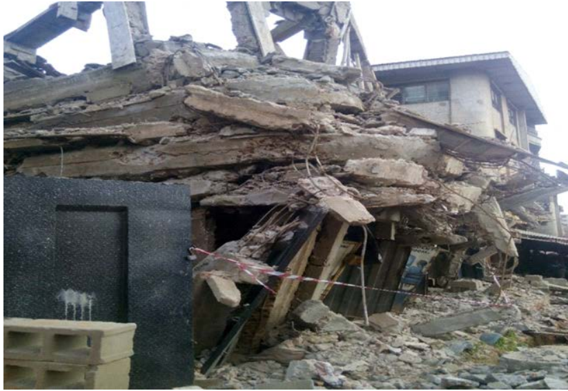
PLATE 1: COLLAPSED 5 STOREY BUILDING AT NO 8 ALLOY OFFIA CRESENT MGBUKA NKPOR ONITSHA ANAMBRA STATE, NIGERIA.
