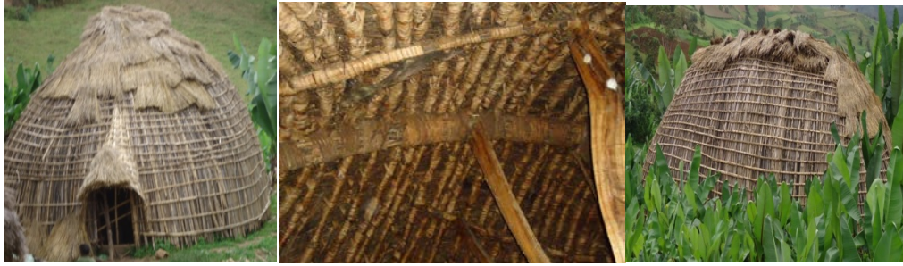
Figure-2.C- Structural view of Waaje type house /from bonke and kucha woredas respectively/
