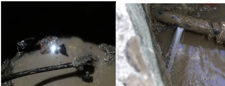
Figure 3: Burst water pipe of supply system
