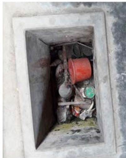
Figure 6: Lack of meter maintenance
