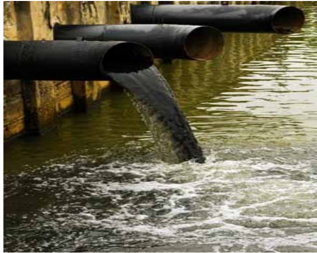
Figure 8: Wastewater discharge directly into water channel without pretreatment
