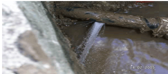
Figure 2: Burst water pipe
