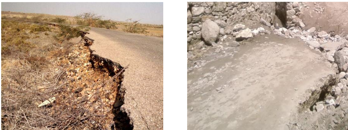
Figure 7: Existing Condition of roads at Gaddani Ship Breaking Industrial Area
