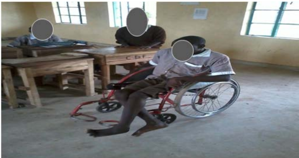
Figure 7: Ample Space provided within the Classroom for Easy Movement of Pupils with Physical disability
