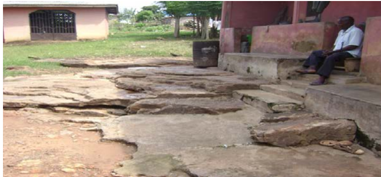
Figure 6: Eroded catchment's top soil exposing impermeable layer in the top soil
